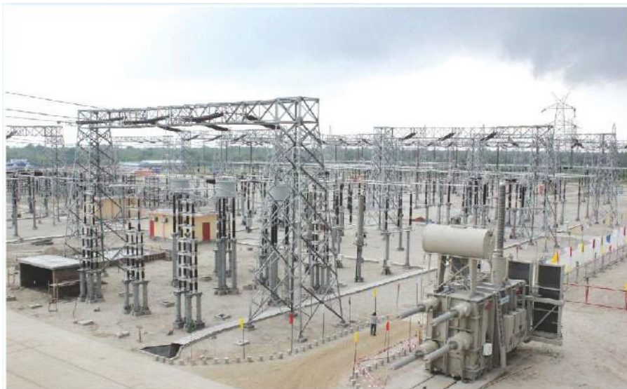
Figure 16: Bangladesh India Power Transmission Plant, Bheramara (Kustia)
