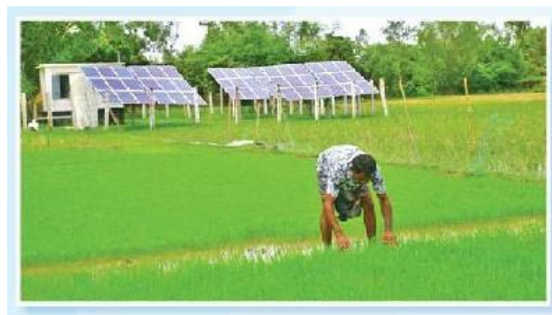
Figure 20: Solar Pump System in Rangpur District
