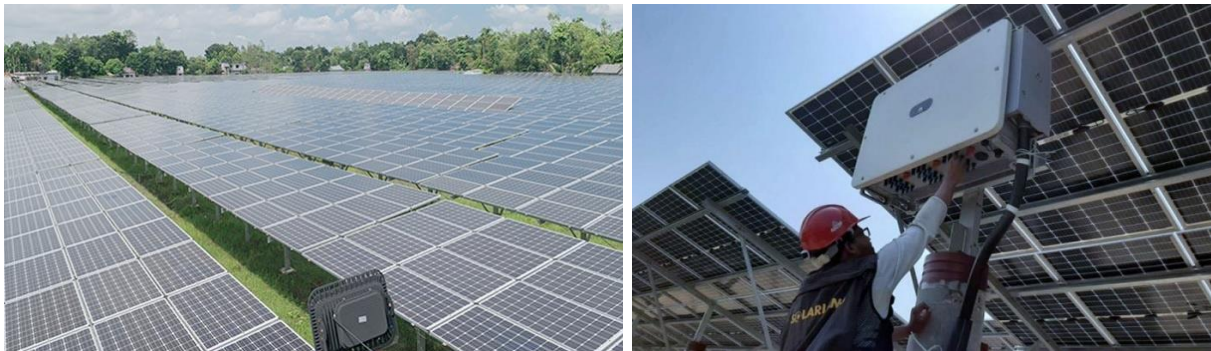
Figure 19: Bangladesh's Largest (73 MW) Solar Power Plant, Mymensingh
