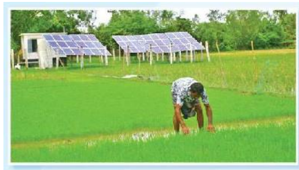
Figure 29: Solar Pump System in Rangpur District
