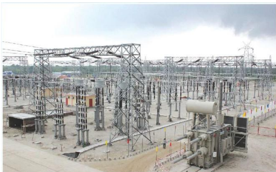
Figure 25: Bangladesh India Power Transmission Plant, Bheramara (Kustia)
