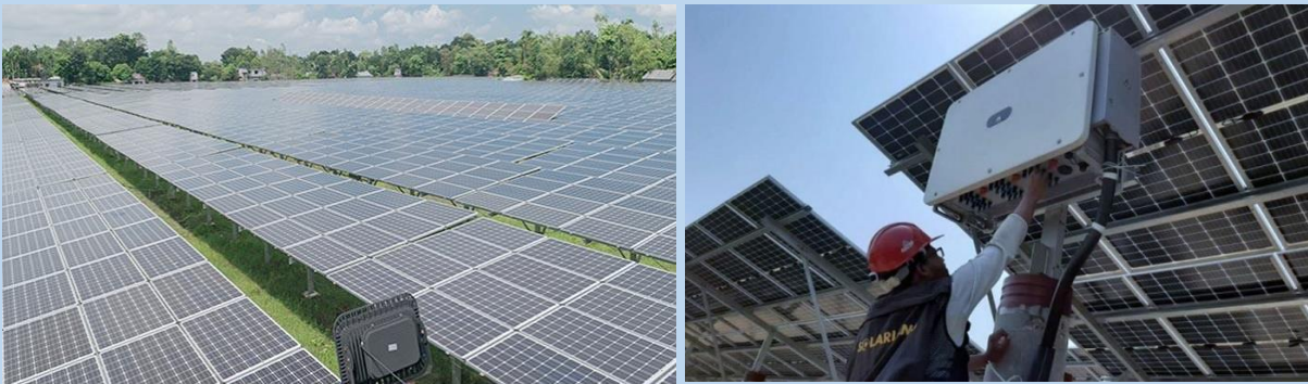
Figure 15: Bangladesh's Largest (73 MW) Solar Power Plant, Mymensingh
