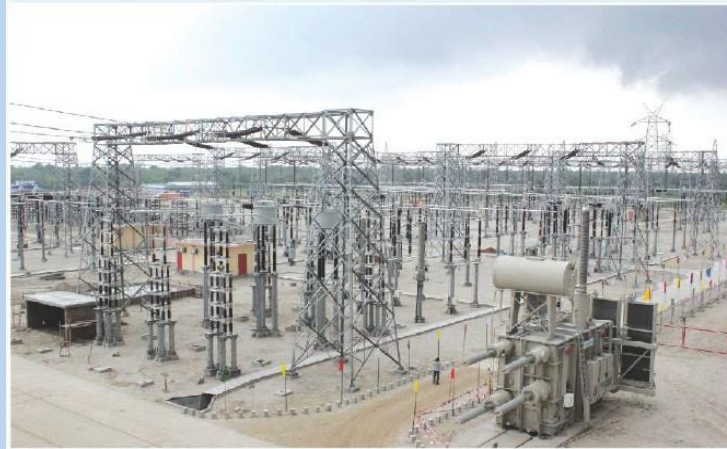
Figure 12: Bangladesh India Power Transmission Plant, Bheramara (Kustia)
