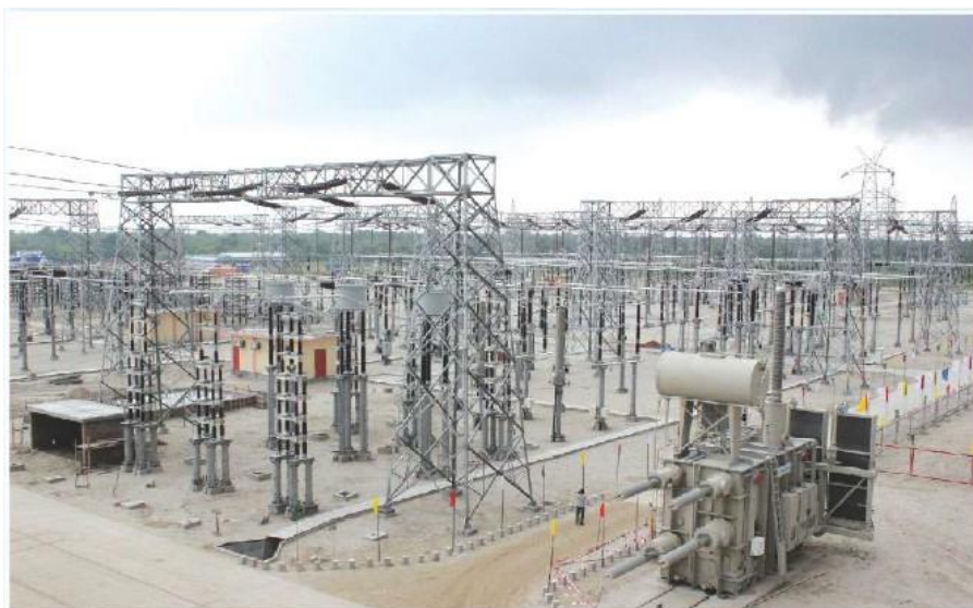
Figure 25: Bangladesh India Power Transmission Plant, Bheramara (Kustia)
